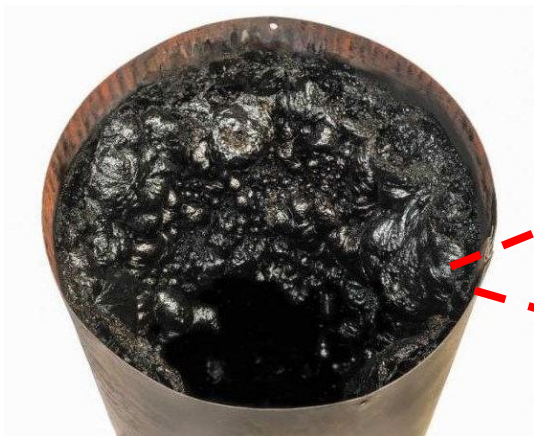
A dangerous creosote build-up in a chimney
