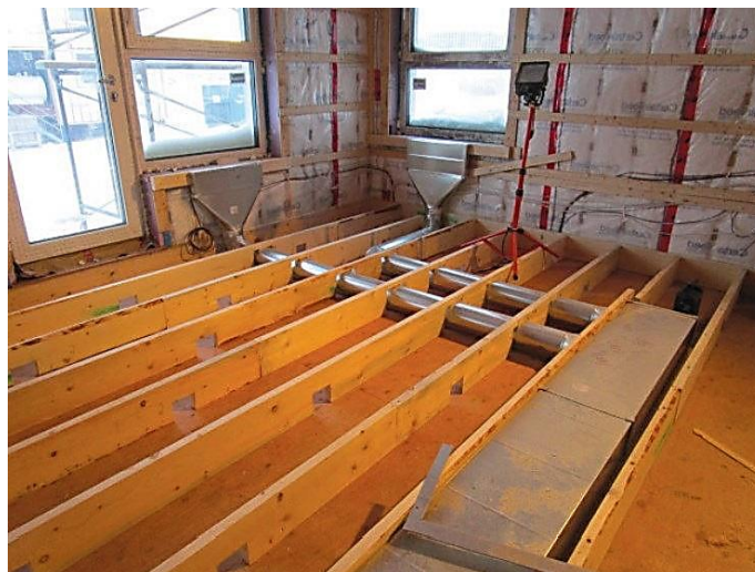
Air-distribution ducting installed in a floor service cavity
