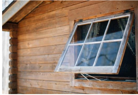
Natural ventilation through an open window
