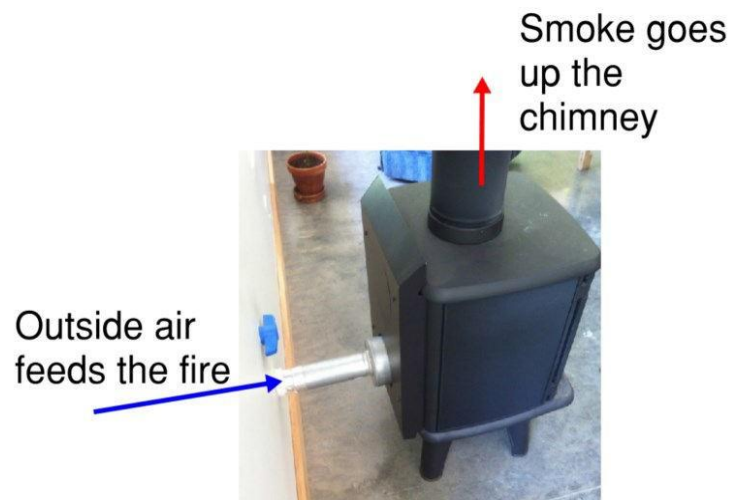
Direct venting of a wood stove with a pipe through the wall
