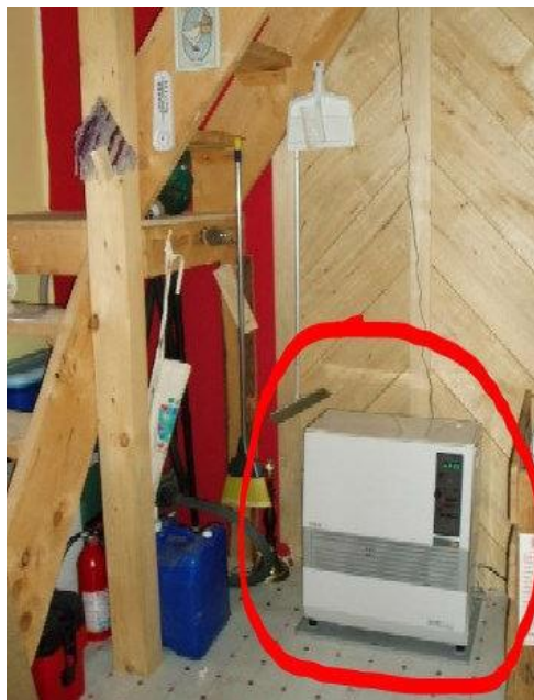
An oil-burning unit heater (Toyo)
