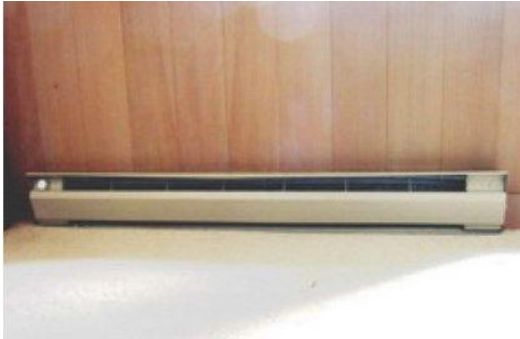
A typical electric baseboard heater that is located in each room of a house.
