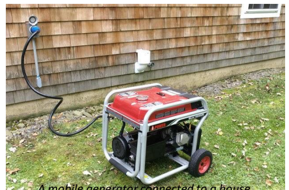
A mobile generator connected to a house
