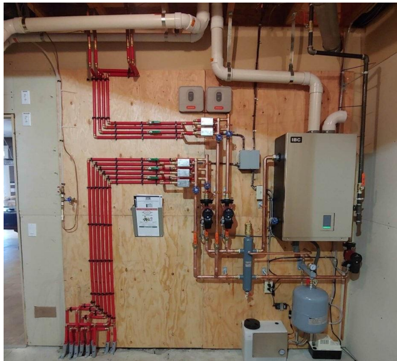
Hydronic boiler equipment with pipe manifold
