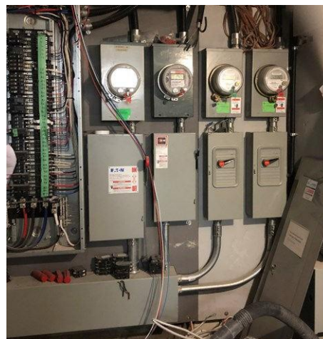
Splitter-feeding multiple disconnects for individual houses
