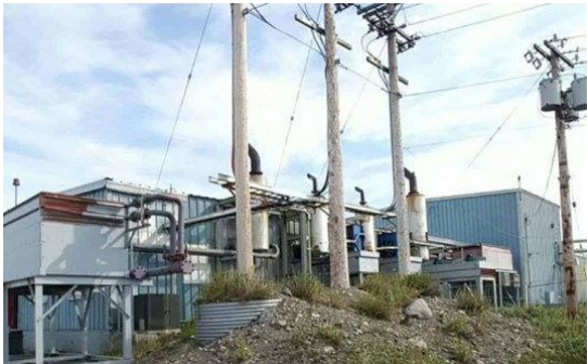
Transformer and Distribution: Overhead power poles
