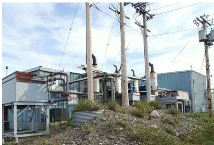
Diesel-generating station with step-up transformers to power poles
