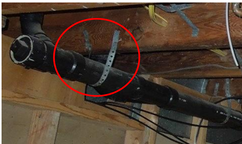
A horizontal pipe supported by a pipe hanger attached to a floor joist
