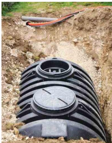
A septic tank
