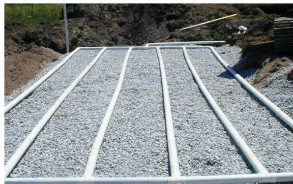
A septic-field installation
