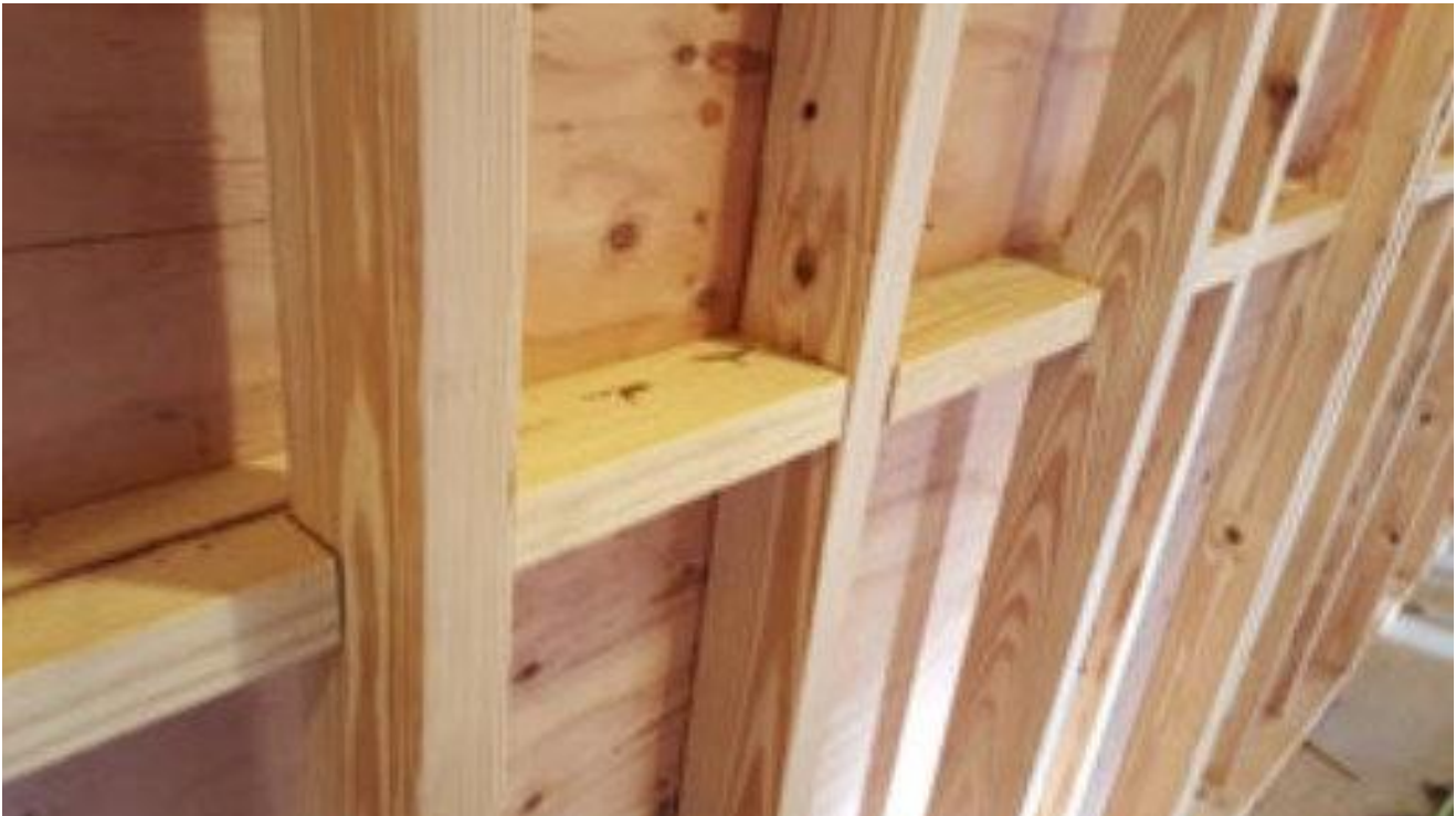
Blocking between studs in an exterior wall to support the horizontal joints in the plywood sheathing
